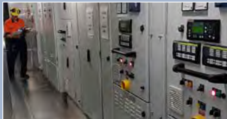
Electrical switchroom installation onboard commercial fast ferry
